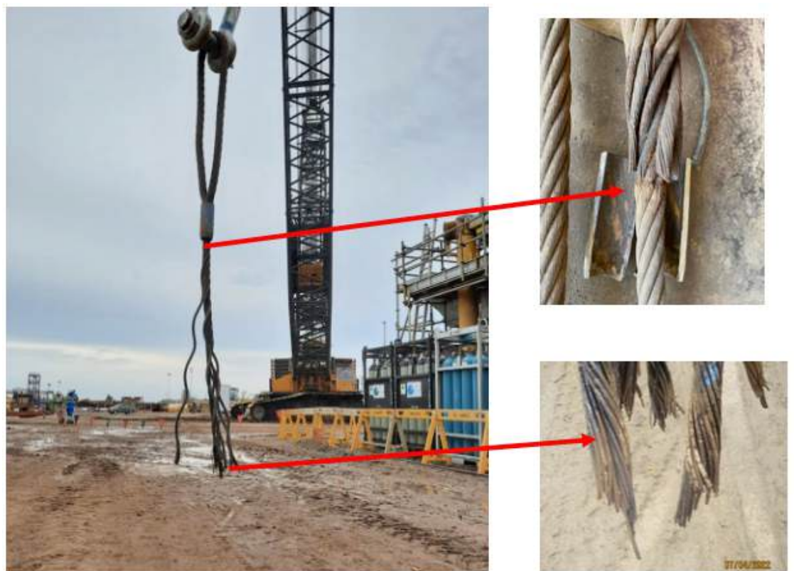
Figure 4. The other end recoiled toward the crane hook. The failure occurred at the sling's ferrule (socket) where the wire rope is swaged, later found to contain corroded wires.
