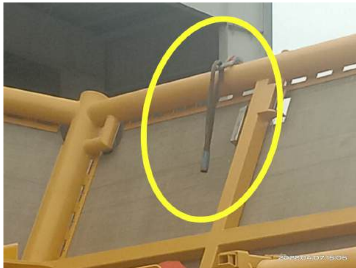
Figure 3. The wire rope sling parted near its end termination – one frayed end remains attached to the panel's padeye (yellow circled).
